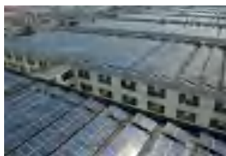
Factory roof solar photovoltaic panels
